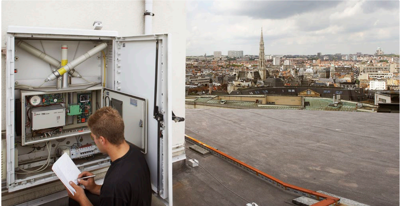
▲ TELERAD measuring station on the roof of the FANC building in Brussels
