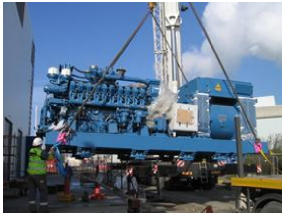
Figure 2 : Installation of the new safety diesel generators in the DGG of units Doel 1 & 2
