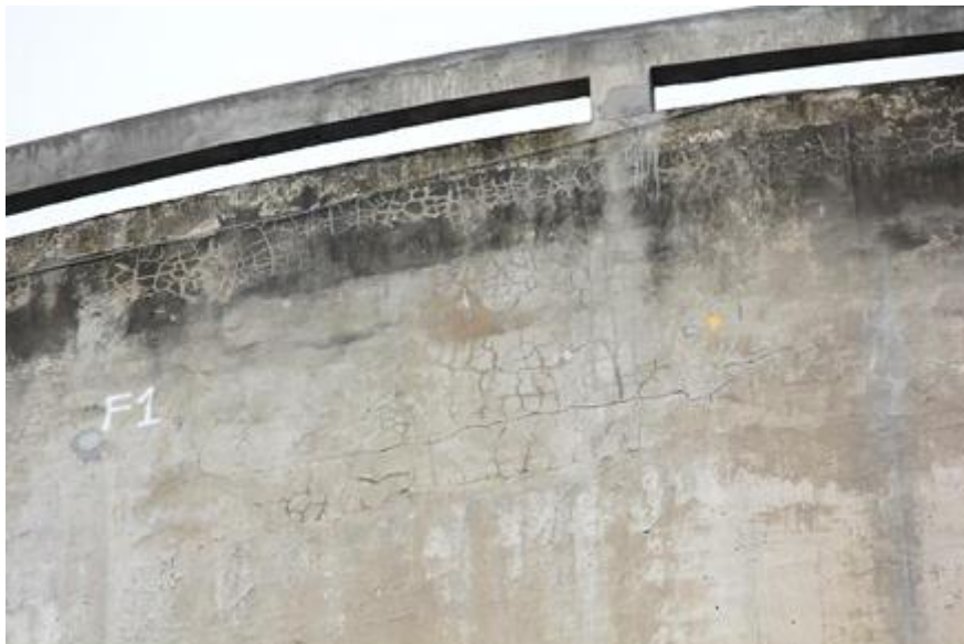
Figure 3 : Zone affected by the alkali-silica reaction (ASR) awaiting repair at the top of the external containment building of Tihange-2 unit (photograph: Bel-V).
